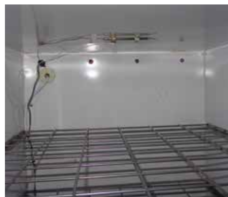
The sensor for the greenhouse controller is mounted to the ceiling inside the kiln. The four holes drilled through the upper back wall of the freezer can be seen.
