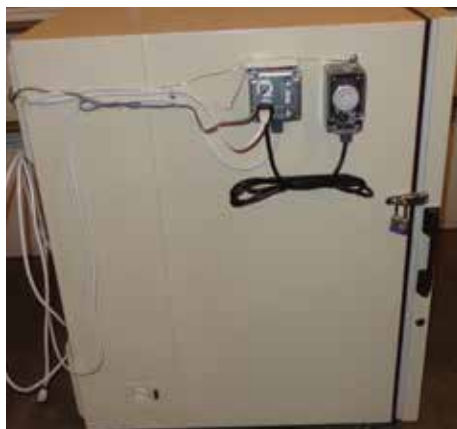
Mounted on the left-hand side of the kiln are the controls, power switch, and outlet, as well as the greenhouse controller. Note the padlock for safety.
